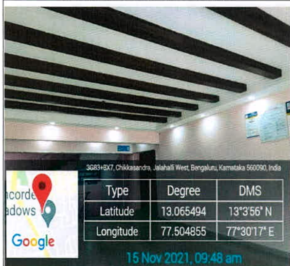
LED fitting in Main Entrance
