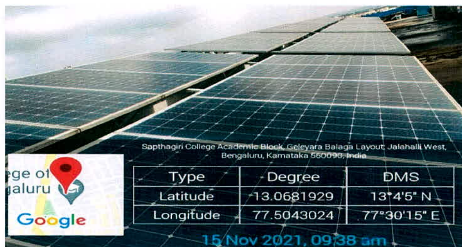
Solar rooftop panel at C- block
